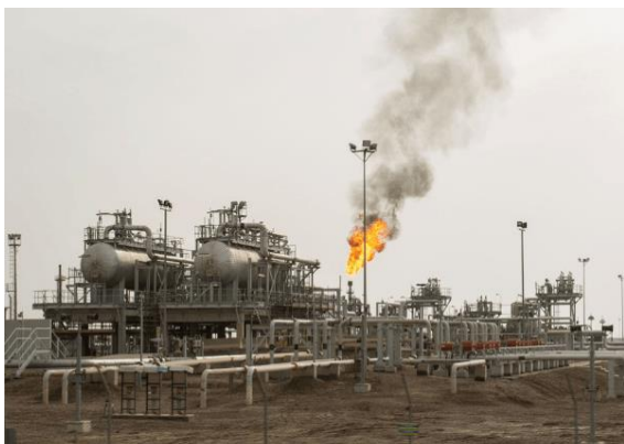
Figure 2: OML-147 Vertical gas flare stack at Owa-Alidinma flow station (Azeez, 2017).
