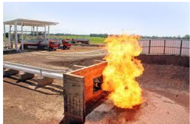
Figure 3: OML-147 Horizontal gas flare stack at Owa-Alidinma flow station (Azeez, 2017).
